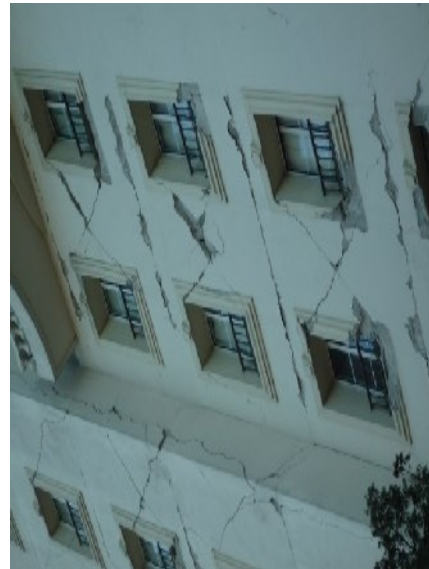
Japanese Embassy in Haiti: Showing Severe Cracks and in Danger of Collapse
